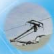
HV connection cables and connectors to carry electricity from the pantograph to the transformer
